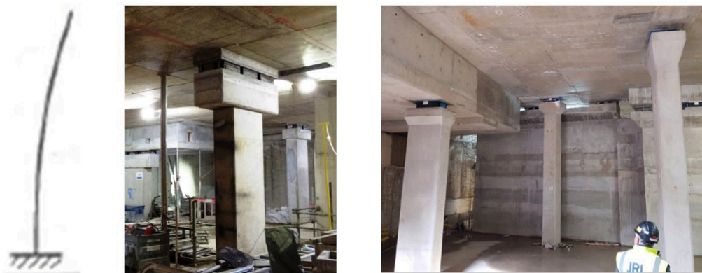
Figure 4: Examples of column bearing assemblies designed with no lateral restraints at the top of columns since they have been designed to have an effective length of x2, concrete column heads, fail safes, vertical continuity ties (left but not required in the right hand photo since there was only one basement level) and a partial full replacement strategy (for example in case of fire)
