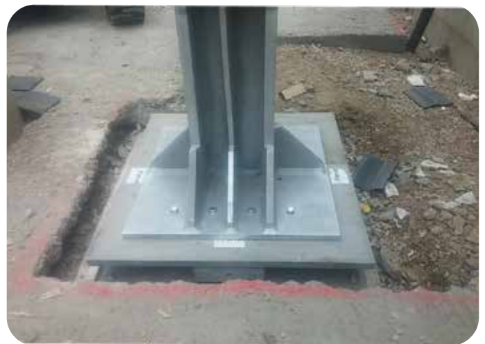
Fig 10.6 Bearing Assembly Supporting an External V Column Integrated lateral restraints withstand lateral forces from the V column as well as a 150 kN force from a potential vehicle impact.
