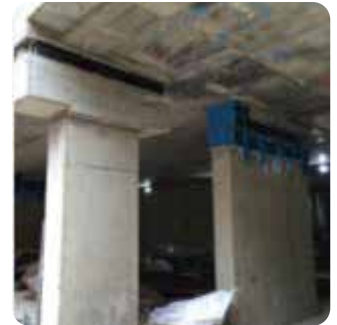
Fig 9.2 Vertical Support Bearings
