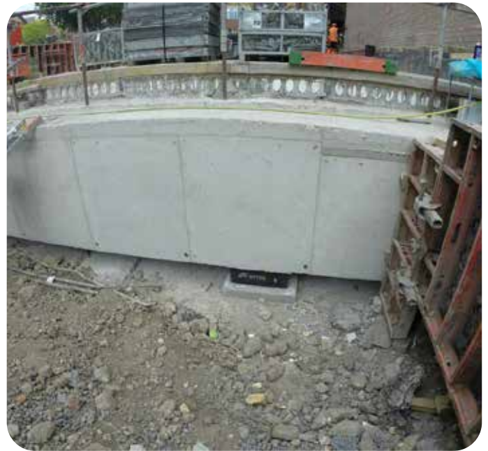
Fig 10.5 Farrat Natural Rubber Laminated Acoustic Bearing This is supporting and isolating the RC ground slab and the precast concrete ground floor slab.
