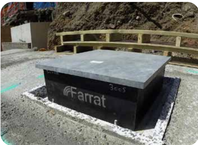
Fig 10.4 Farrat Natural Rubber Laminated Acoustic Bearing This is grouted in place with a galvanised levelling plate below and galvanised formwork plate above, ready for the RC ground beam formwork to be constructed around it.
