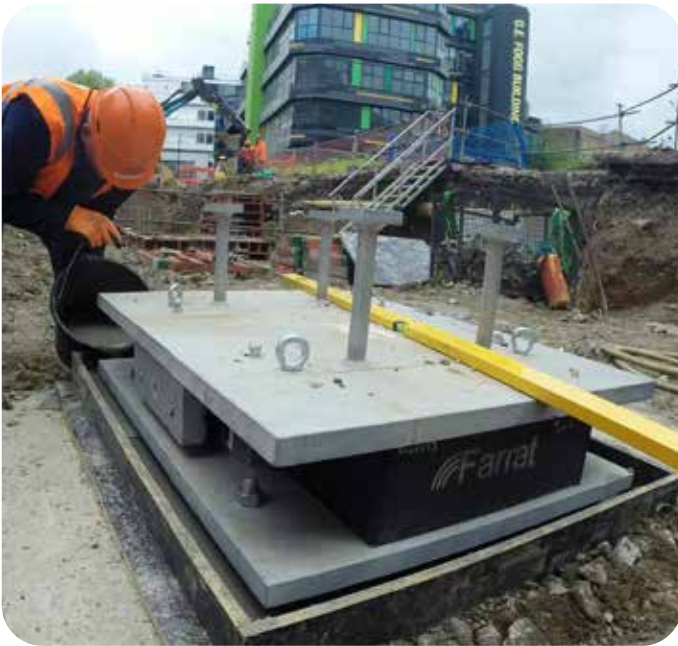
Fig 10.3 The Lateral Restraint Bearing Assembly During Installation Care was taken throughout the grouting process to avoid air pockets within the grout bed.
