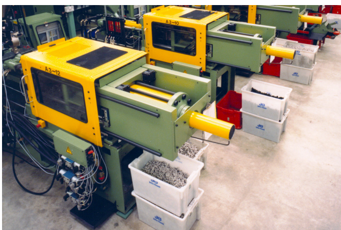
Fig. 1.1 Injection moulding machines installed on Farrat Isomounts
